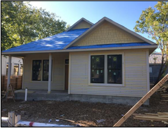
This home features cement board siding with a 4" reveal which mimics the appearance of wood siding.
